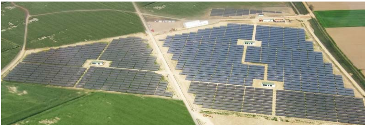
6MW of Kyocera modules at Enermill's solar power plant in Cigliano, Italy
